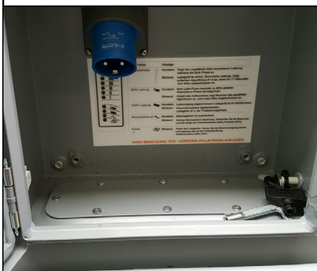
Fig 37: Match the correct voltage charger to the port.
