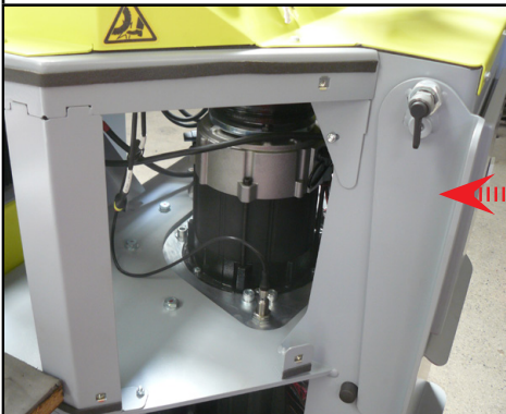
Fig 33: Cover removed from ED.
