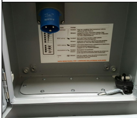
Fig 20: Match the correct voltage charger to the port.
